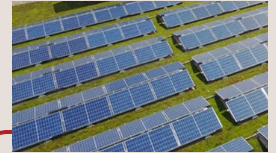
Solar Panel in Roof area
