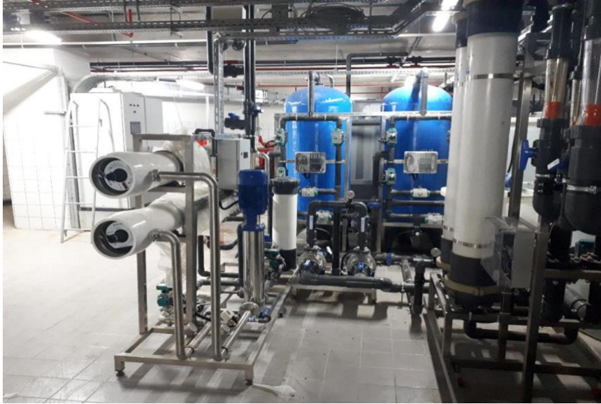
Greywater Microfiltration system
