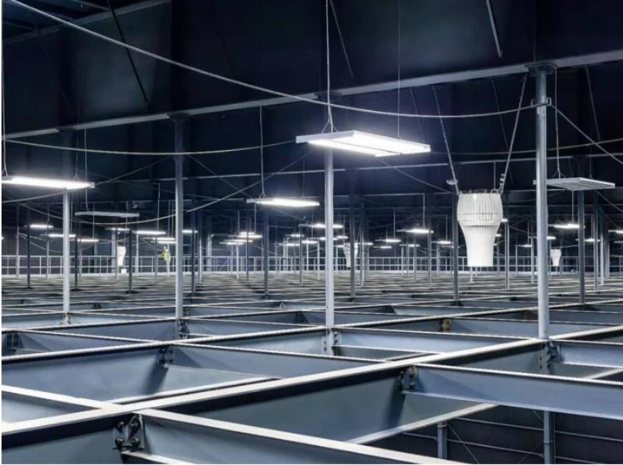
Figure 24: Destratification Fans Installed under Ceiling
