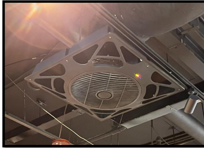
Figure 39: Hybrid Cooling Aircon and Fan at SDC
