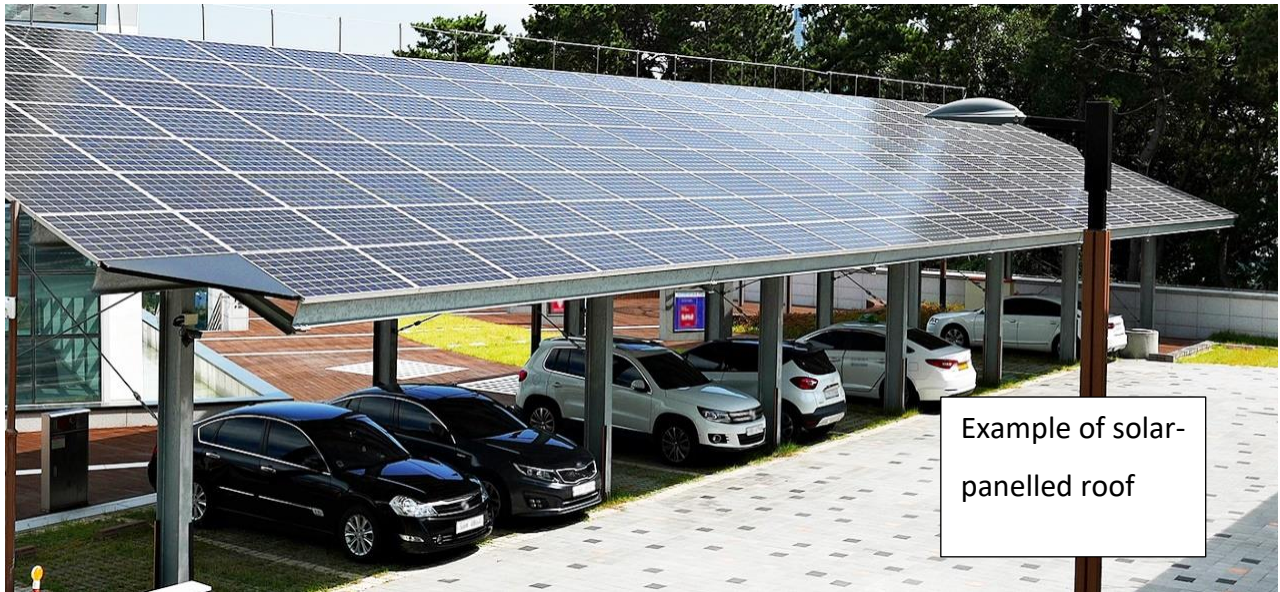
Figure 6: Solar-panelled roof (Megawatts, n.d.)
