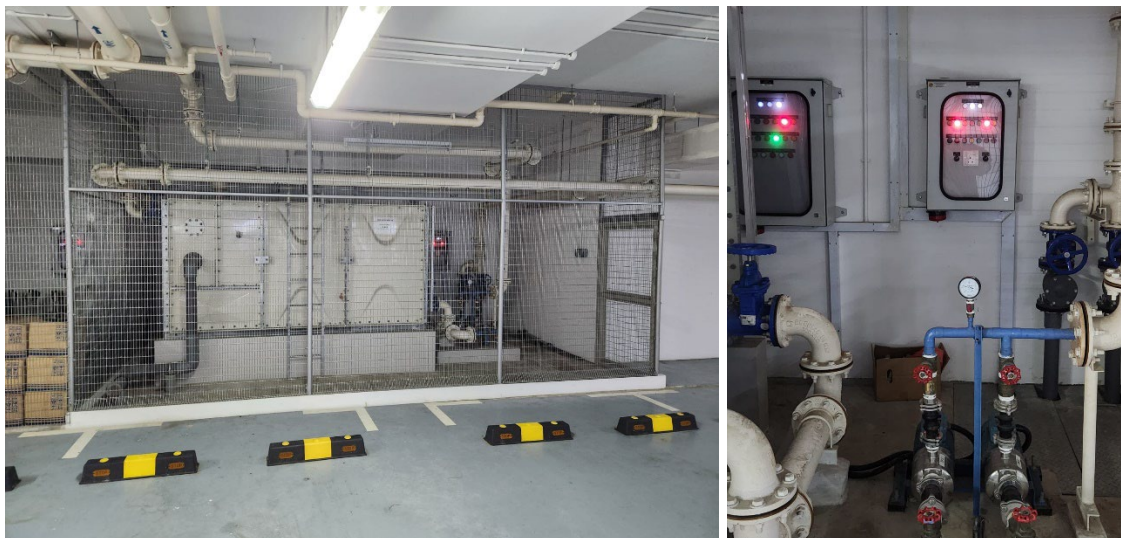
Fig 2.31: Basement transfer water tank and transfer pump
