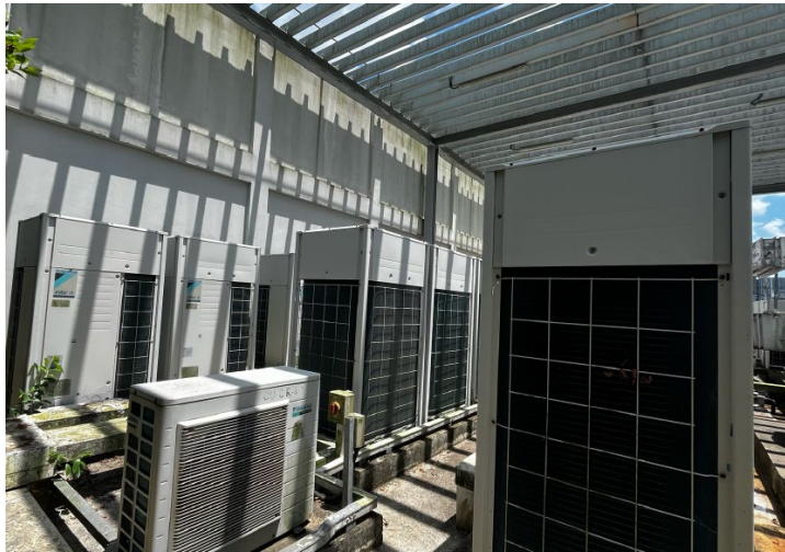
Fig 1.322: Exiting older generation VRV-IV in rooftop
